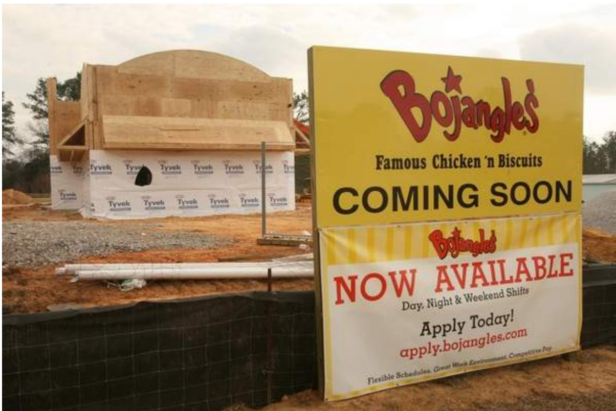
(Michael E. Palmer/Tuscaloosa News) Staff photo | Michael E. Palmer A Bojangles' restaurant is being constructed in Northport.
